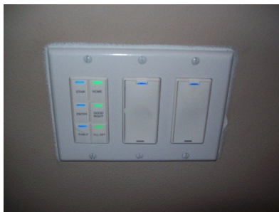
Programmed light switches
