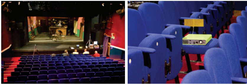
Figures 25 and 26: The ADC auditorium and a Neul WSD, in situ Photos: Les Smith
