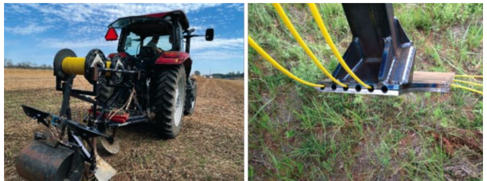
A specially designed plow system to install FO-DTS cable with minimal soil disturbance.
