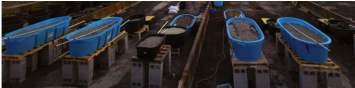
Six pilot-scale, three-stage hybrid constructed wetlands installed by an ECU Capstone engineering senior design team at the Greenville Utilities Commission wastewater treatment plant in Greenville, North Carolina.
