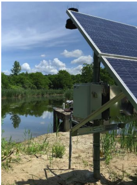
A solar-powered stormwater control panel that uses cloud-based real-time control software.
