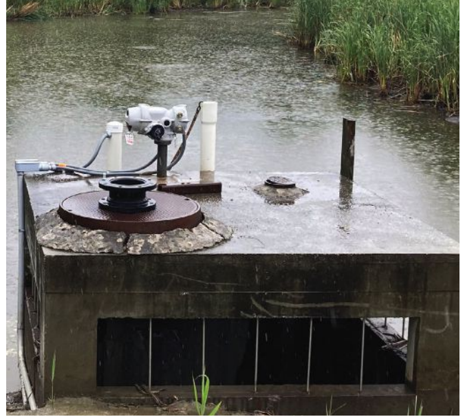
A stormwater control structure with a remotely actuated valve for automated real-time control.
